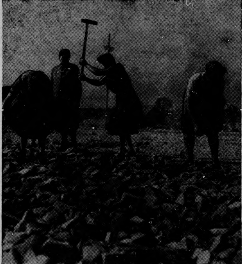
HELP ALLIED AIRLIFT . . . In order to increase the potency and efficiency of the Allied airlift into beleaguered Berlin, more air strips had to be built. Scores of German women, like those pictured above, are aiding the Allies by helping to build a new runway at Tegel, in the heart of the French sector of Berlin. These new strips relieve the heavy burden from the Tempelhof airport.
