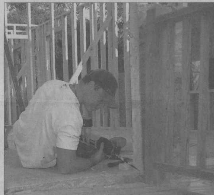
Jason Bliss, a volunteer worker with Habitat for Humanity, constructs a door frame on the house being built this week on Greene Street. PHOTO BY CANDI HAUGLUM
