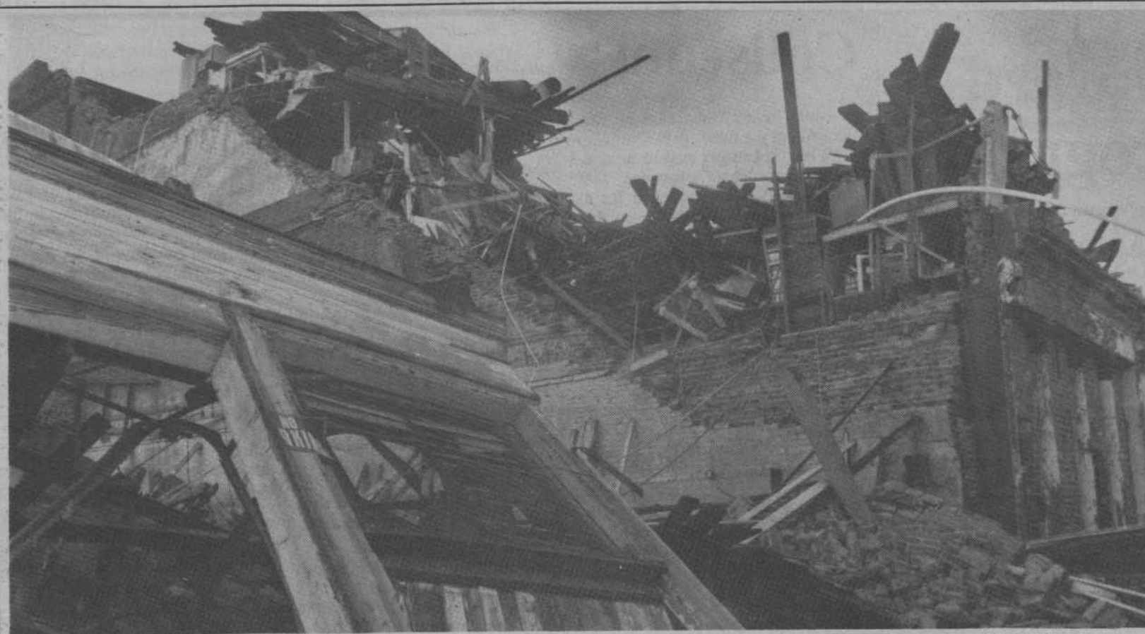
This building on King Street in Charleston, where the historic horse-drawn carriages were kept, displays the destruction Hurricane Hugo left in its path as it ripped along South Carolina's coast Thursday.
