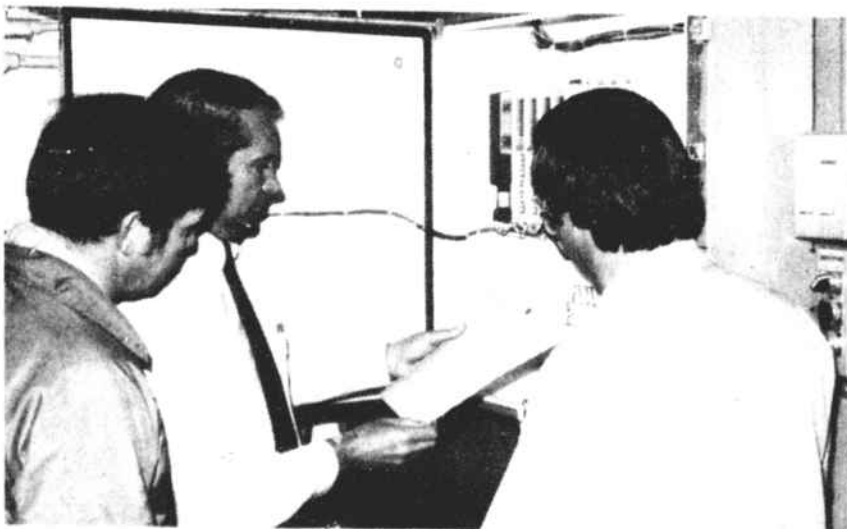
MICROPROCESSOR FOR NO. 1 —Assistant Plant No. 1 and 2 Engineer Johnny Price, Director of Plant Engineering Silas Campbell and Marshall Vaughan, note the computer technology that has been brought to the No. 1 plant as this device greatly improves the handling of stock between the various departments.
