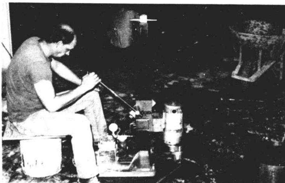
EXISTING FLOOR CLEANING ENLARGED —Al Reid Construction Company is working rapidly to enlarge the existing floor cleaning openings so that this work can be completed before each unit of looms arrives.
