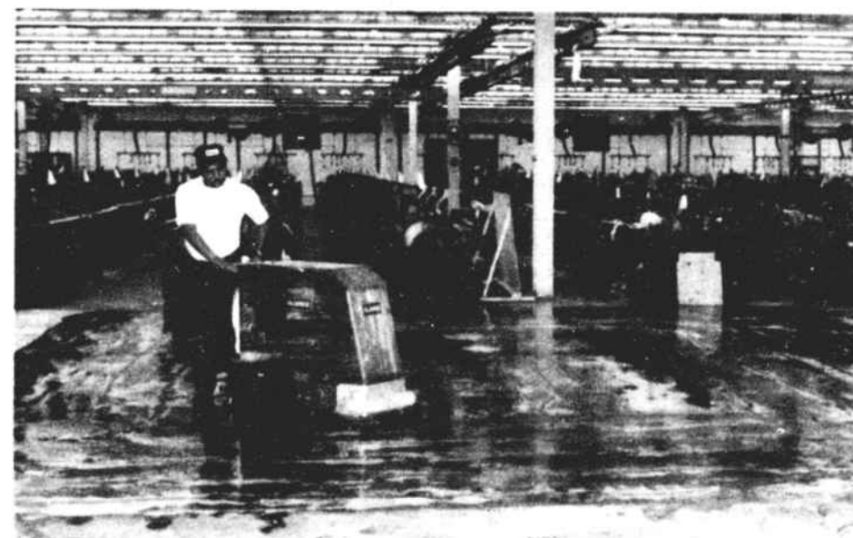
FLOOR SCRUBBING A NECESSITY —Much emphasis is being placed on keeping the Bailey Plant clean and orderly during the renovation process. As an area is completed, it is prepared for the arrival of various pieces of new equipment.
