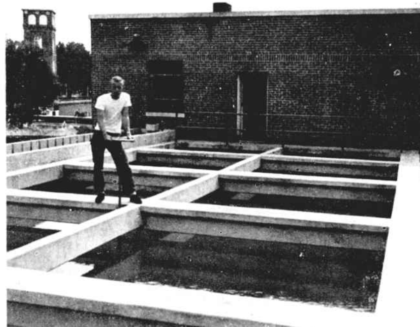
THESE SETTLING TANKS at the Clinton-Lydia filter plant are the first step in purifying the water you drink, use in the mill and in the pools, is purer than the highest state standards.
